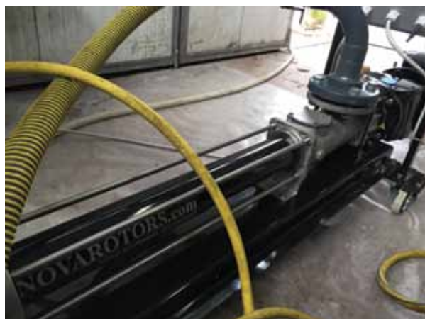
Fig. 6 - Detail of the hydraulic system used to transfer the ELS® concentrate from the drum to the mixing tanks and from the mixing tanks to the injection point.
