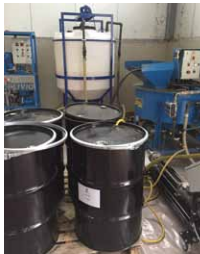
Fig. 7 - Pre-mixing tank (on the right) and final mixing tank with in-line recycling system (in the middle).
