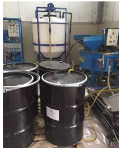
Fig. 7 - Pre-mixing tank (on the right) and final mixing tank with in-line recycling system (in the middle).
