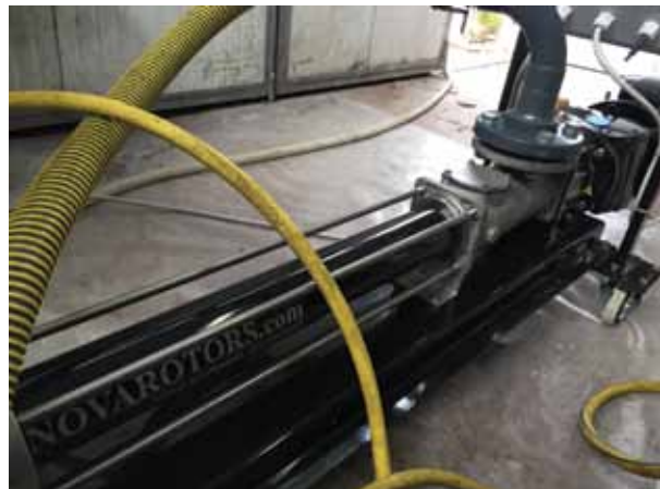
Fig. 6 - Detail of the hydraulic system used to transfer the ELS® concentrate from the drum to the mixing tanks and from the mixing tanks to the injection point.
